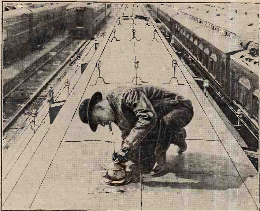
TWO-WAY TELEPHONY ON TRAINS. Wired-wireless is now used on the Canadian National Railways to enable passengers to converse with telephone subscribers in the principal cities. The photograph shows the antenna system on the Toronto-Montreal express.
